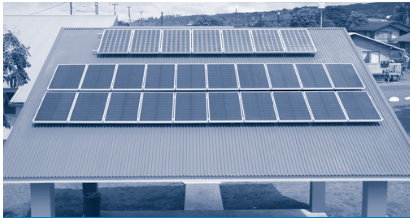
These solar-electric installations at Lanai High and Elementary School sit atop a new, outdoor gathering area. The performance of two types of panels will be compared to see which is better suited to capture the sun's energy in cloudy locations.
